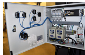
Control Panel Design/Build
